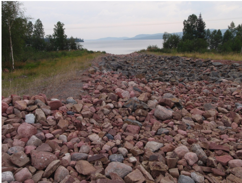
Photo 6: Photo of armored spillway constructed to improve land bridge stability (looking towards Beaverlodge Lake)
