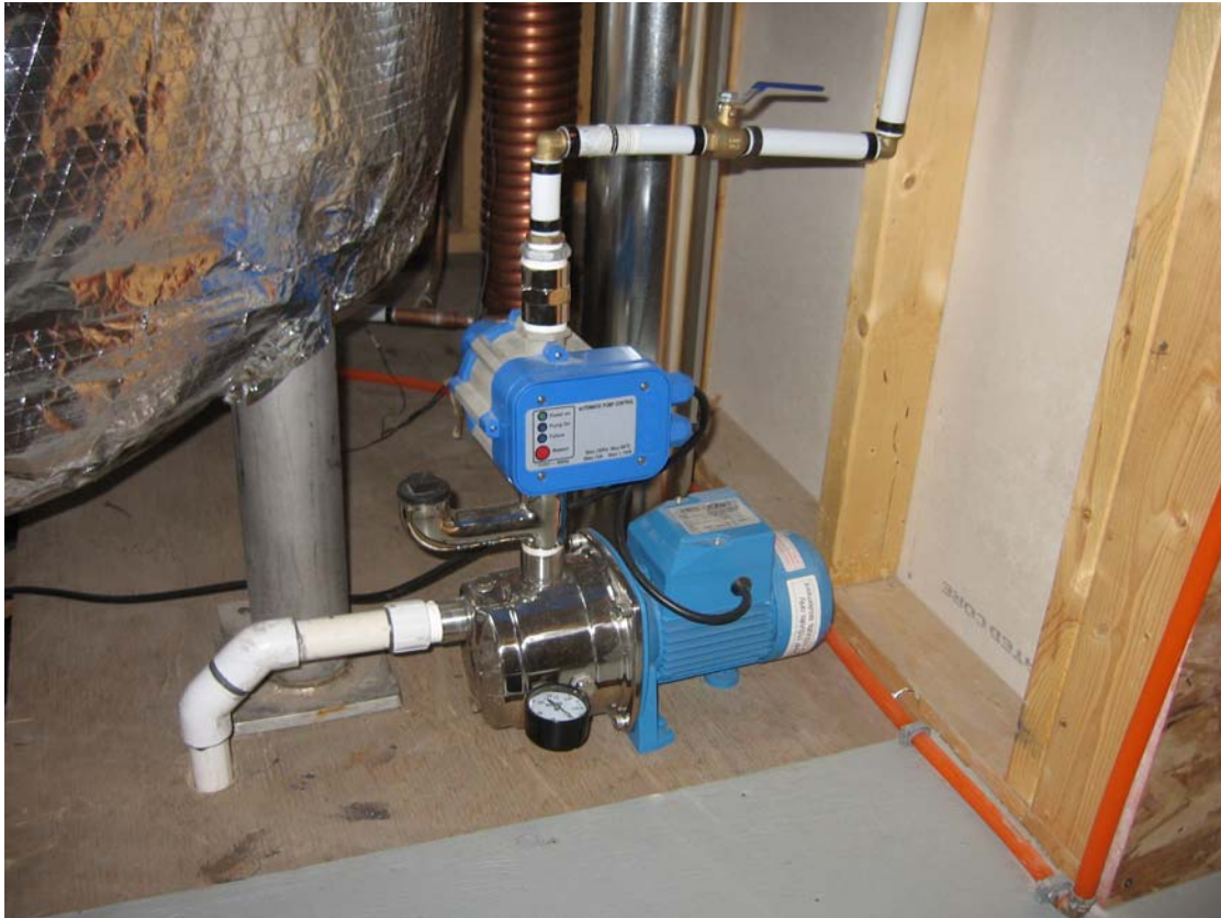
Figure 22: Water pump to supply the toilets and the exterior landscaping
