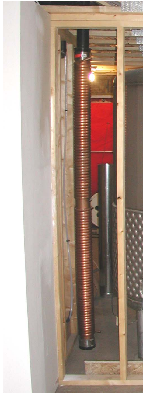
Figure 18: Copper waste water heat exchanger for the house
