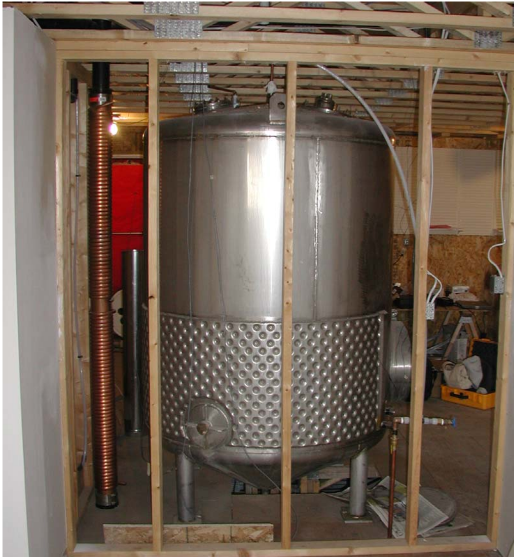
Figure 16: Stainless steel heat storage tank
