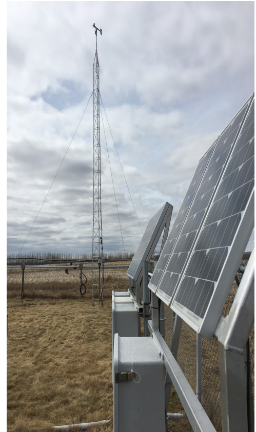
Anemometer tower 25 March 2017 photo: R. Jansen
