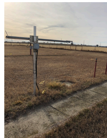
Snow Depth Sensor maintenance Nov 2020 Photo: V. Wittrock
