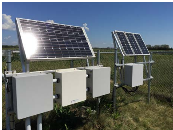
Data loggers and communication 28 June 2016 Photo: R. Jansen
