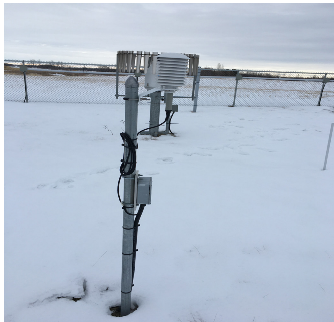
Air Temperature Sensor January 2018 Photo: Development Engineering and Manufacturing
