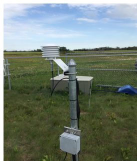
New air temperature sensor August 2018 Photo: Development Engineering and Manufacturing
