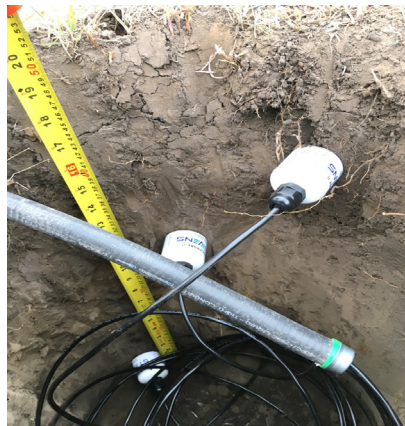
New Soil Moisture Sensors installed 24 Oct 2018 October 2018 Photo: K. Babich
