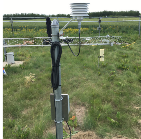
New Air Temperature Sensor Aug 2018 Photo: Development Engineering and Manufacturing
