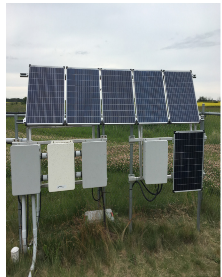
Increased solar power. July 2019 Photo: Development Engineering and Manufacturing
