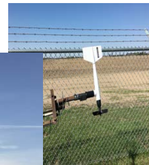
RM Young Wind Speed & Wind Direction ready bearing replacement May 2017 Photo: R. Jansen
