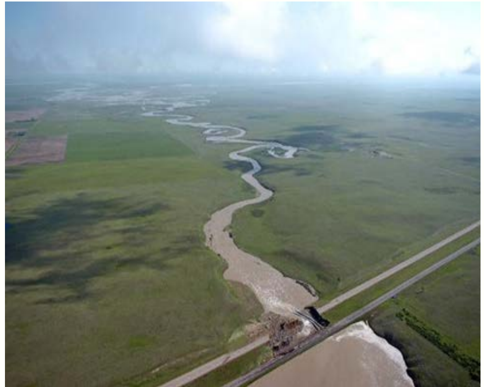
Photo: WSA, TransCanada Highway washed out June 2010
