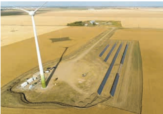
1,400 solar panels were added to the Cowessess Energy Storage Facility in 2018.
