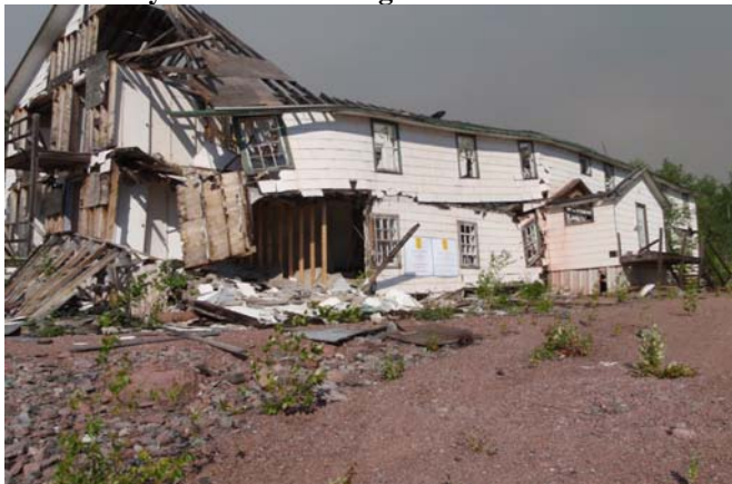
Structurally unsound building
